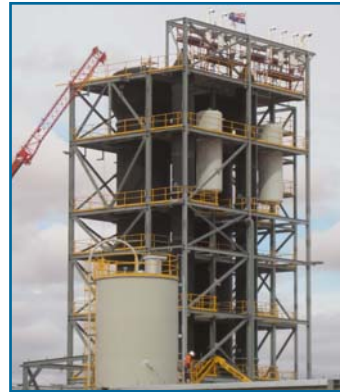
Honeymoon solvent extraction (February 2010)
